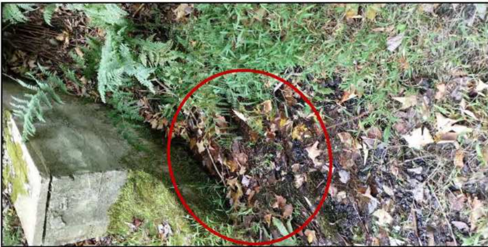
Photo 2 – Seep just downstream of dam.
