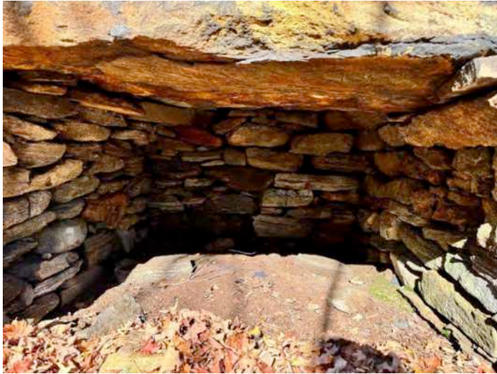
Mysterious hole in the face of the dam.
