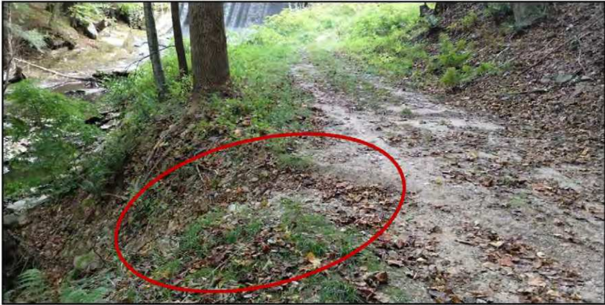
Photo 12 – Erosion on access road. Looking northward towards the dam.
